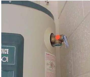
(Fig.1) TPR Valve with no discharge tube
